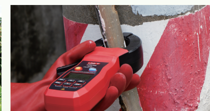
Measurement of Transformer Ground Resistance
